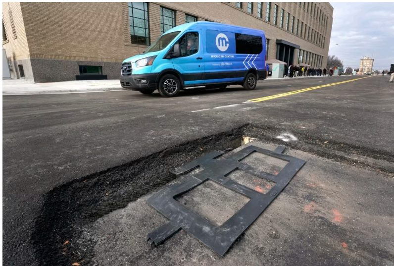
An in-road wireless charging coil before being installed in a street in Detroit in 2023. PHOTO: PAUL SANCYA/ASSOCIATED PRESS
